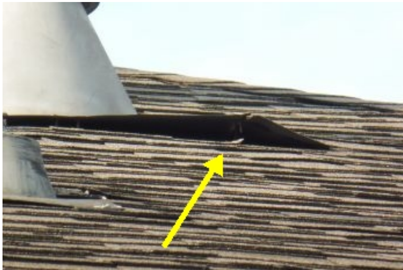
Lower side of flashing is not sealed down at one or more locations. wind driven rains may allow water penetration.
