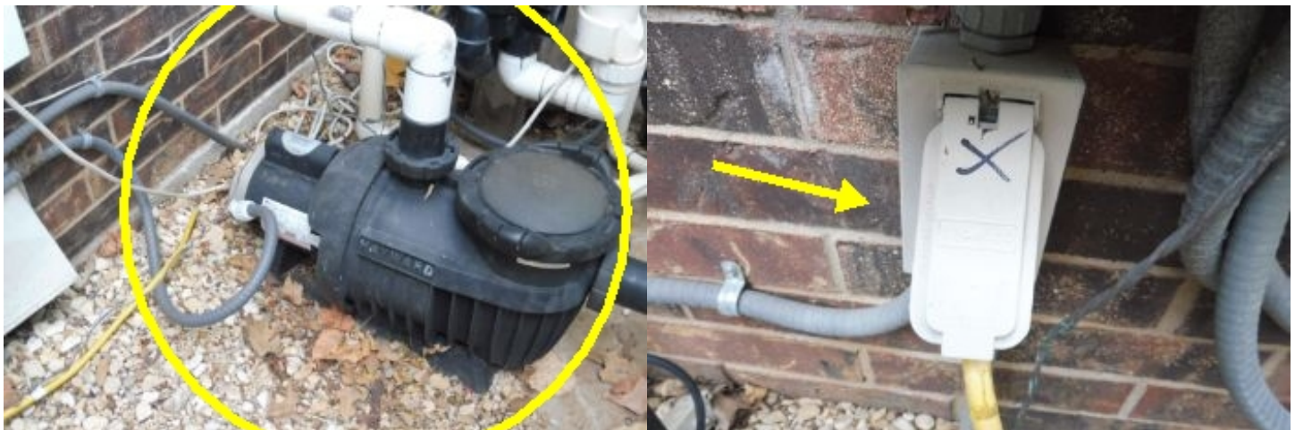
Water leaks were observed in the area of the pool motor/s and equipment and should be repaired.
