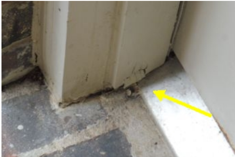
Wood rot or other damage appears present at the bottom of one or more exterior door frame areas.
